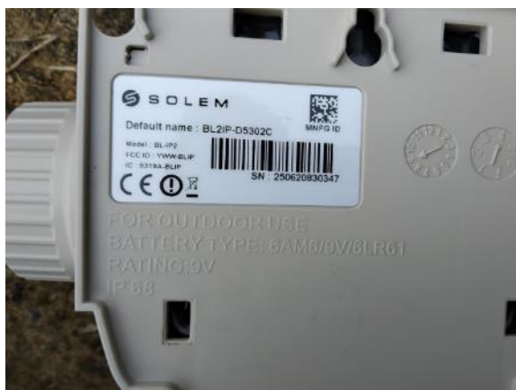
Garden Pictures - Next to Mailboxes Phase 6 Olive Trees (replacing broken Rain Bird programmer with 1 Solem 2E)
