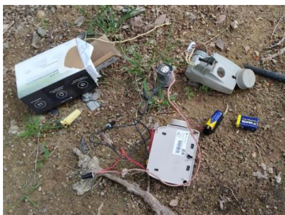
Garden Pictures - Vandalism: 2 programmers ripped out (Rain Bird programmer replaced with Solem)
