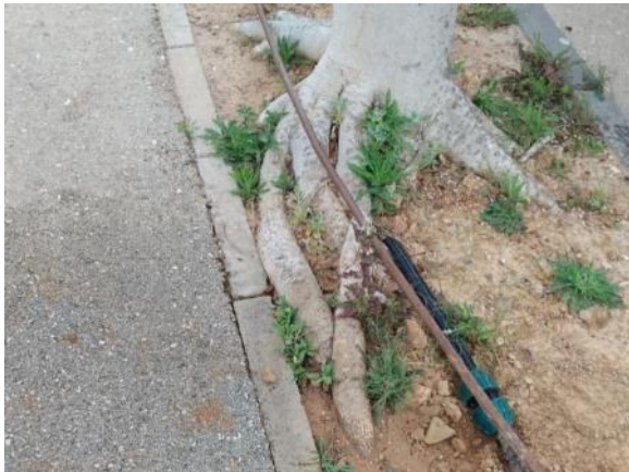
Paseo Alameda (Oasis) - End next to new buildings (50 ml PE Ø16, 1 link)
