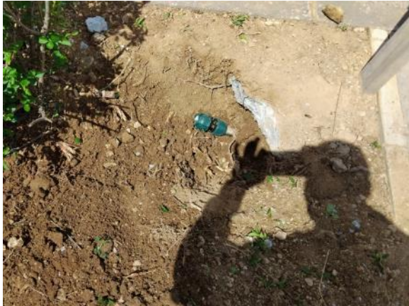
Main vial - Root damage in front of Hotel (35 ml PE Ø32, 3 links)
