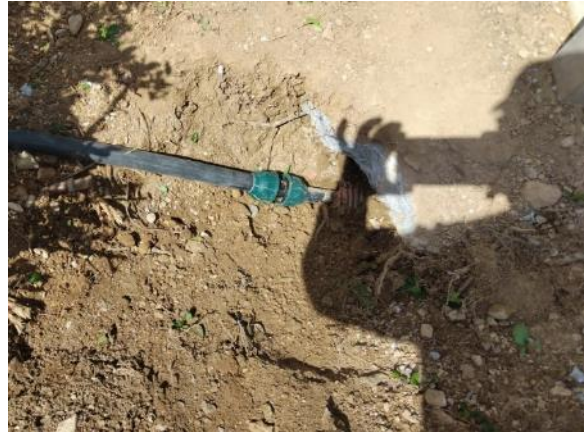
Main vial - Root damage in front of Hotel (35 ml PE Ø32, 3 links)
