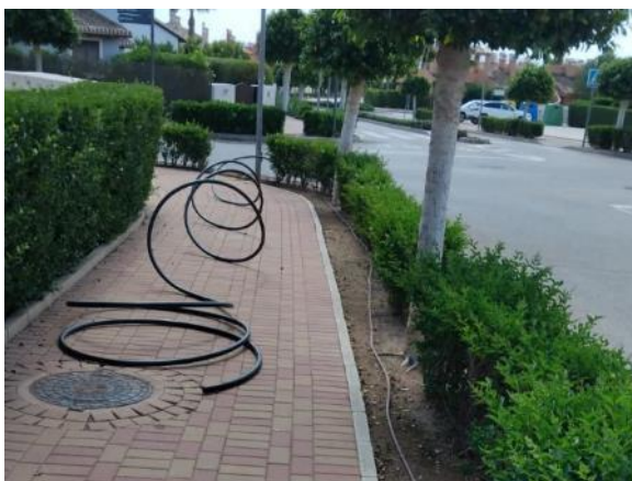
Main road - Flowerbed next to the Clubhouse parking lot (replacement 58 ml PE Ø16, 4 connections)
