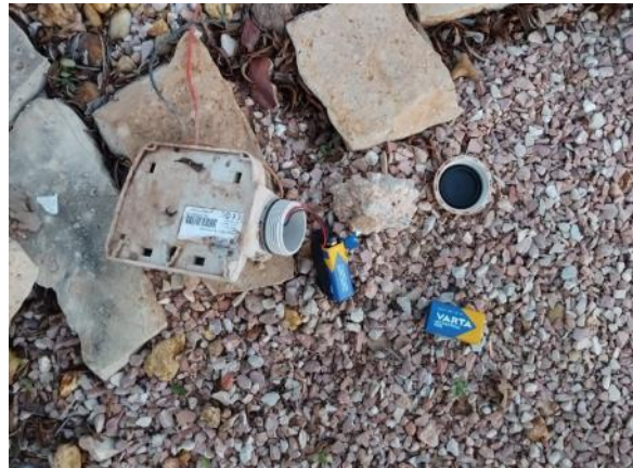
Phase 2 - C/ Bahamas (programmer battery replacement)
