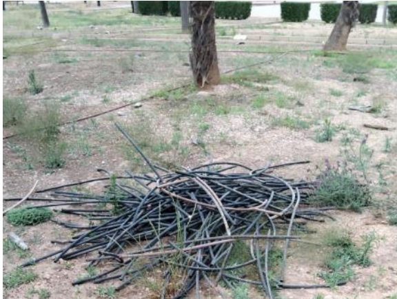
Garden behind the Security Guards - Drip line refill (180 ml PE Ø16, 44 drippers)
