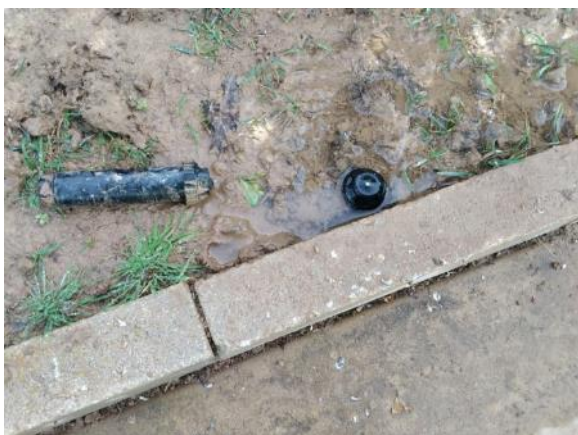
Cuadros Garden (next to Olivos mailboxes) - Replacement of broken diffuser
