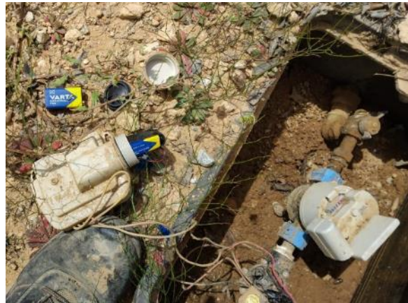
Los Olivos - Back garden (timer battery replacement)
