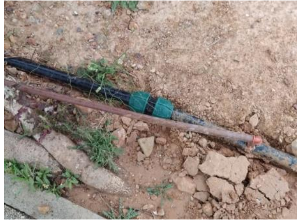
Paseo Alameda (Oasis) - End next to new buildings (2 ml PE Ø32, 1 link)
