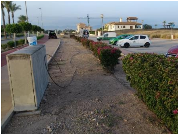
Main road - Flowerbed next to the Clubhouse parking lot (replacement 58 ml PE Ø16, 4 connections)
