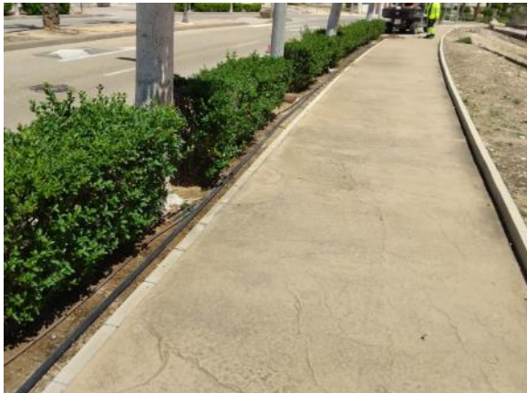
Main vial - Root damage in front of Hotel (35 ml PE Ø32, 3 links)
