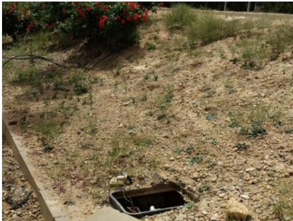
Los Olivos - Back garden (timer battery replacement)
