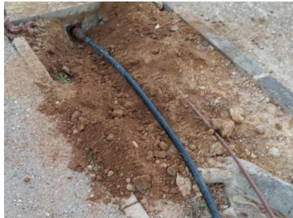
Paseo Alameda (Oasis) - End next to new buildings (50 ml PE Ø16, 1 link)
