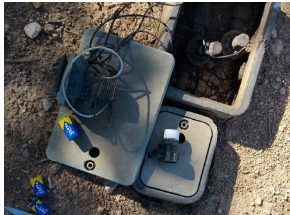
Phase 6 - Olivos B (change of Rain Bird programmer to Solem 2E, 2 solenoid valves and 3 9V batteries)
