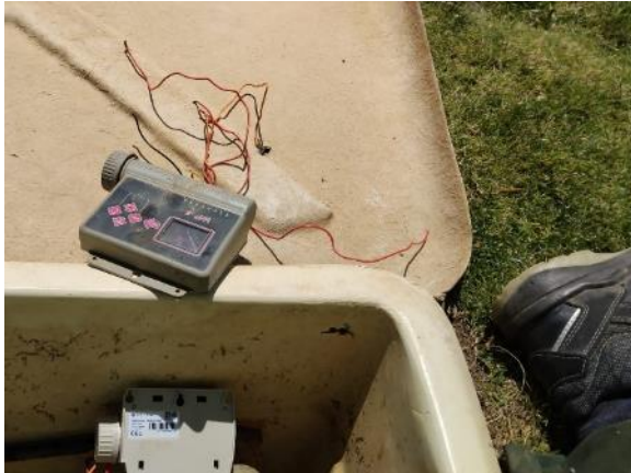
Main Road (entrance) - Olivo Roundabout (change Rain Bird 4E programmer for a Solem 4E and 1 9V battery)
