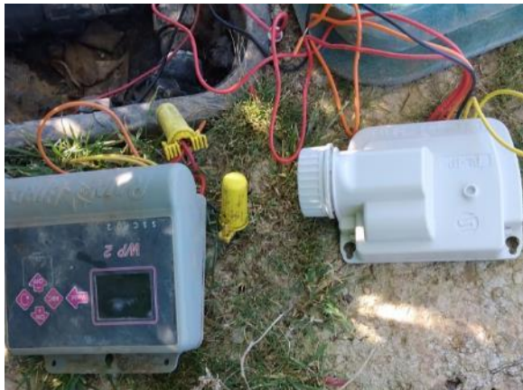
Entrance - Garden by Squares (replacement of 1 Rain Bird programmer by Solem 2E)
