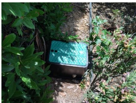
Entrance - Garden by Squares (replacement of the rest of the garden with 7 new SOLEM programmers)
