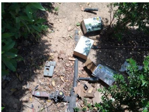
Entrance - Garden by Squares (replacement of the rest of the garden with 7 new SOLEM programmers)
