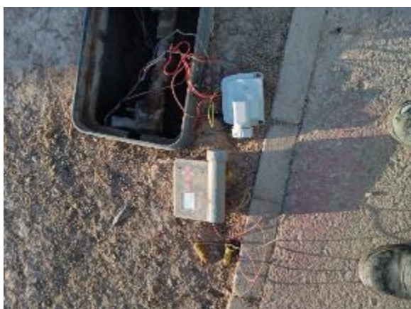
Main Road - between Olivos and EUM (replacement of 1 Solem 2E programmer)
