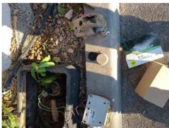
Phase 1 - C/ Germany (replacement of 1 Solem 1E programmer)
