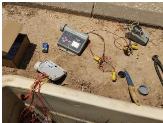
Main road (median) - opposite football field (replacement of 1 Solem 4E programmer)
